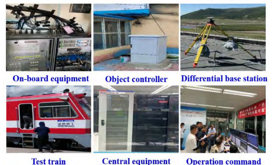
Fig.2. Whole-set system field installation and deployment in HMR.
